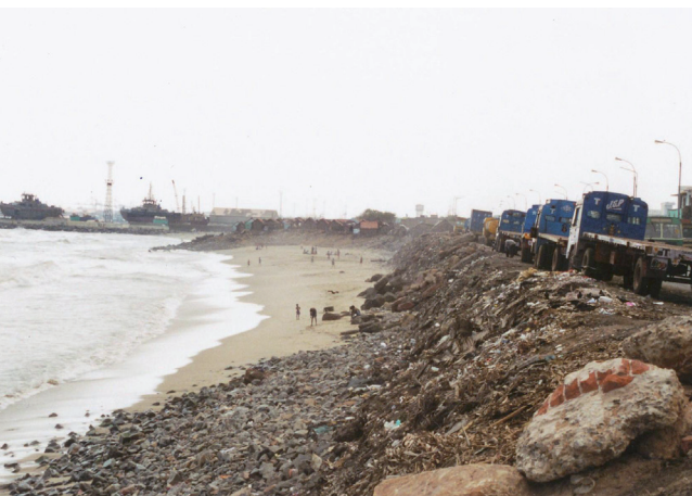
Severe coastal erosion affecting the coastal road, north of Chennai, Tamil Nadu, India. (photo: R. Misdorp)
